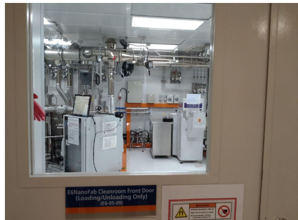
Fig.2 A part of clean room (Campus facility).
